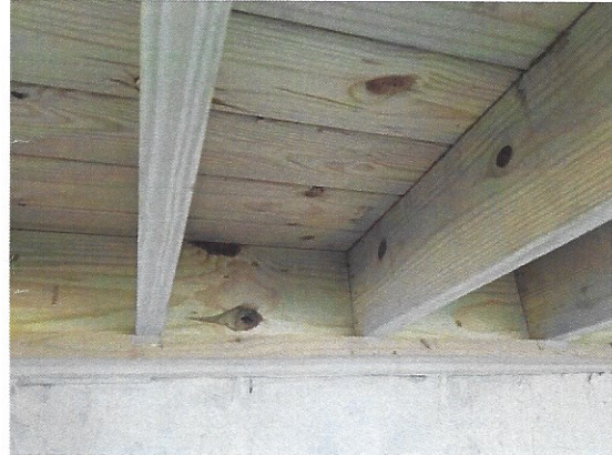
Picture 8 – Example of inadequate attachment of new deck rim band to existing rim bands
