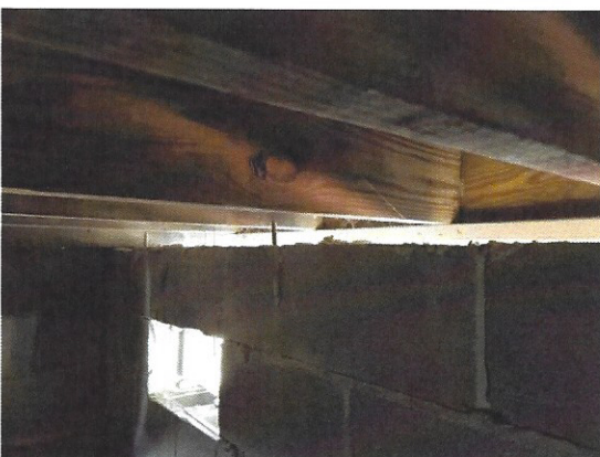
Picture 5 – Example of misplaced foundation wall below screened in porch
