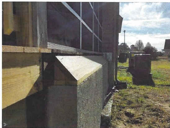
Picture 4 – Example of misplaced foundation wall below screened in porch
