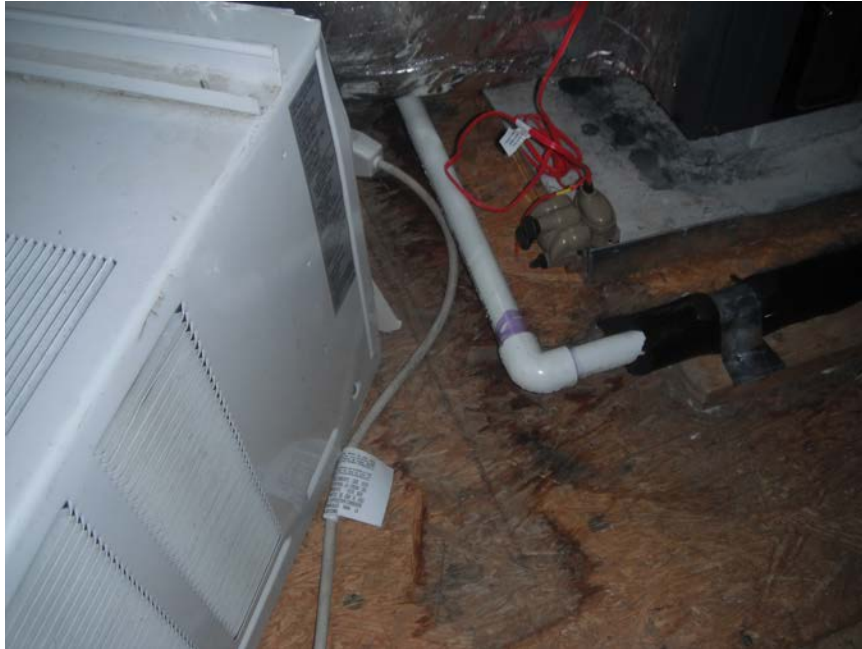
Photograph Number 29 - View of condensate line leak in the attic
