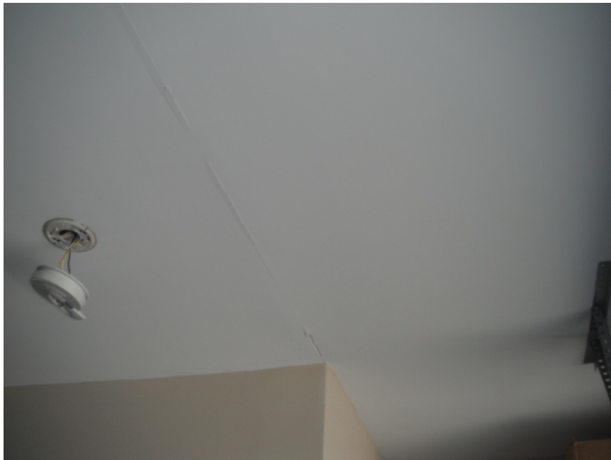
Photograph Number 22 - View of interior drywall crack.
