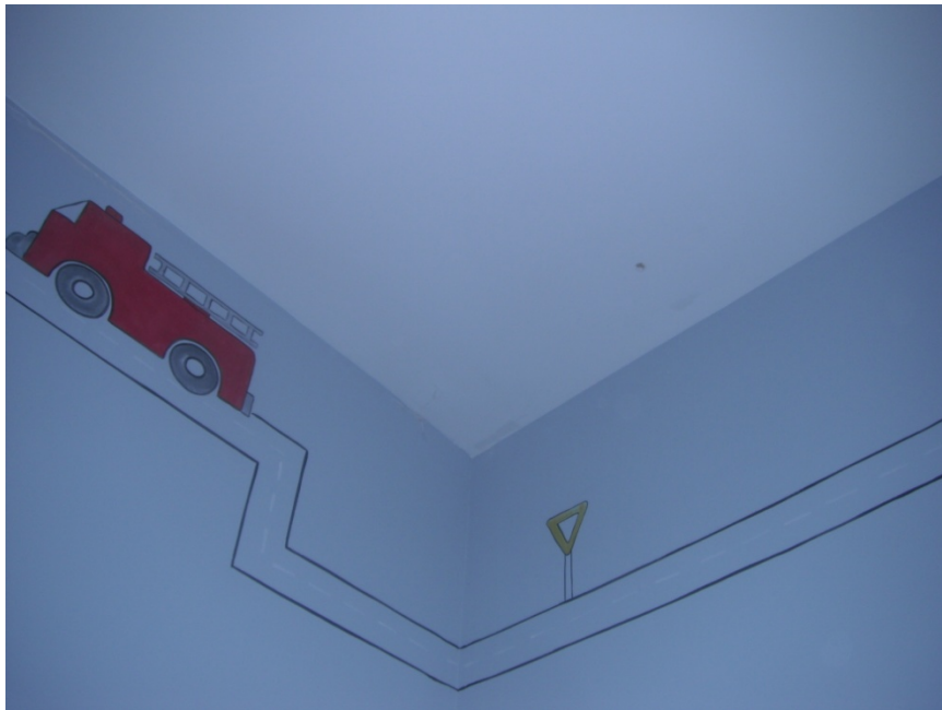
Photograph Number 24 - View of isolated drywall nail pop
