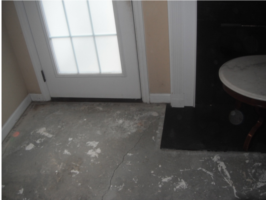
Photograph Number 11 - View of slab cracking at rear chimney area.
