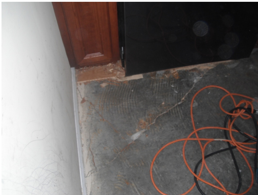
Photograph Number 14 - View of slab cracking.
