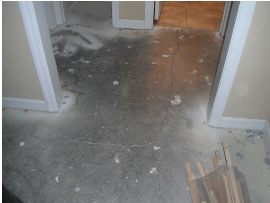
Photograph Number 12 - View of slab cracking.
