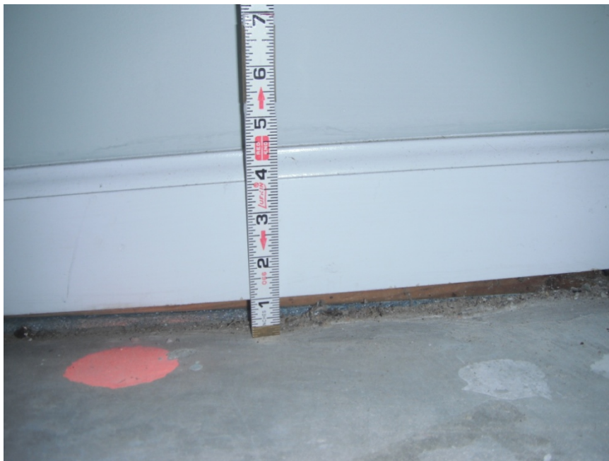
Photograph Number 18 - View of separation between slab and wall framing
