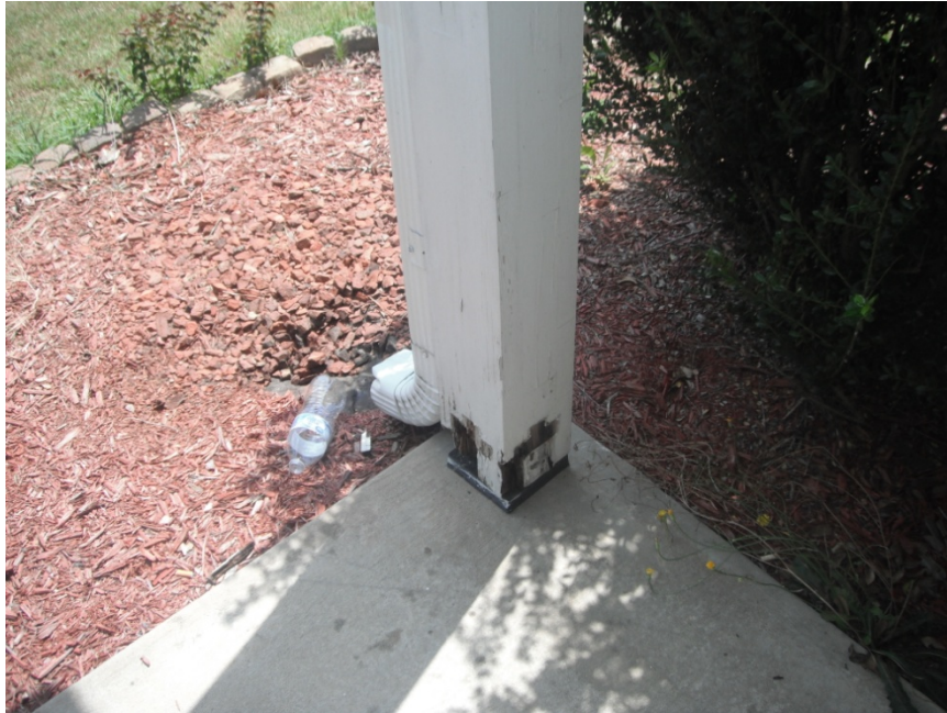
Photograph Number 27 - View of deterioration at front porch corner post
