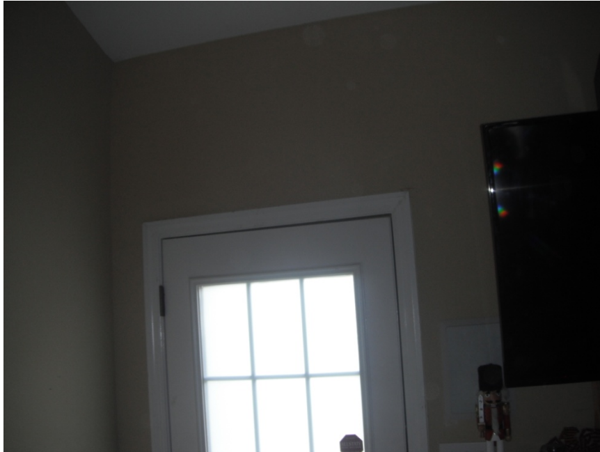
Photograph Number 21 - View of rear entrance door misalignment
