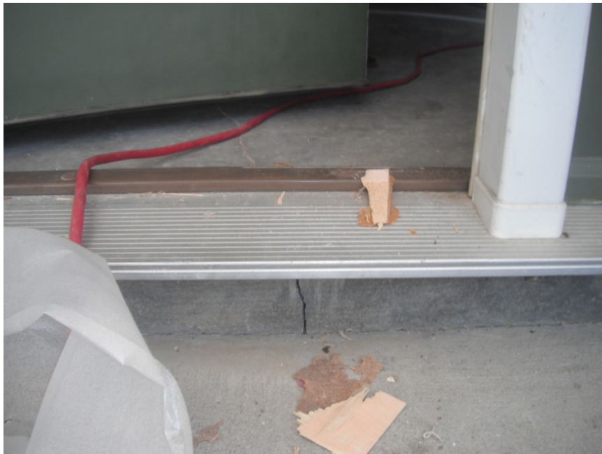
Photograph Number 6 - View of slab crack located below front entrance door
