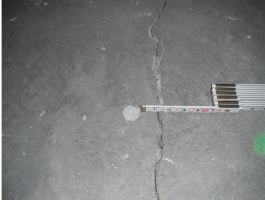
Photograph Number 15 - Close up view of slab cracking.
