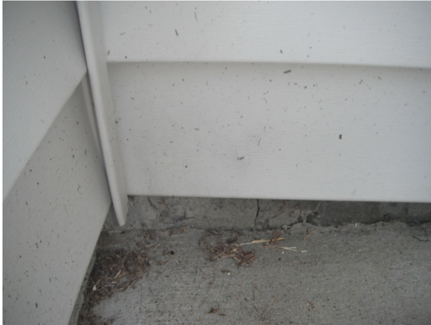
Photograph Number 9 - View of slab crack - rear exterior
