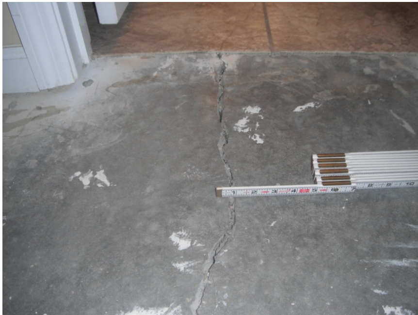
Photograph Number 16 - Close up view of slab cracking.
