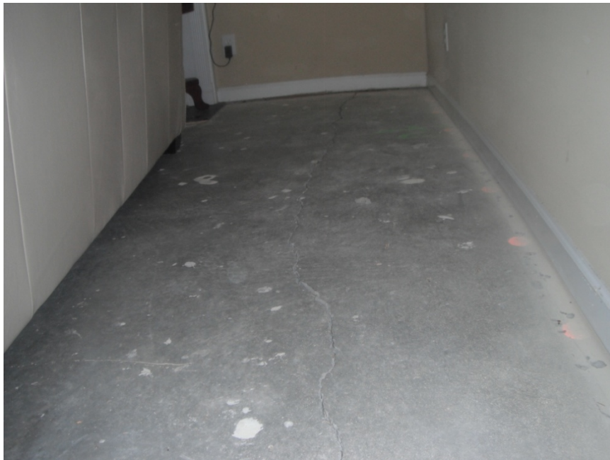
Photograph Number 10 - View of slab crack extending front to rear in living room area.
