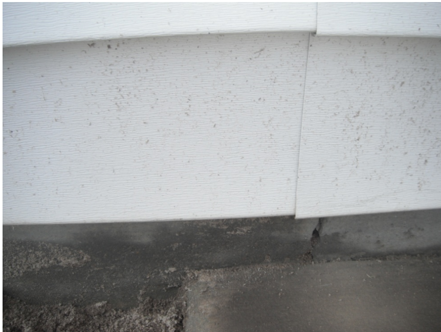
Photograph Number 8 - View of slab crack - rear exterior
