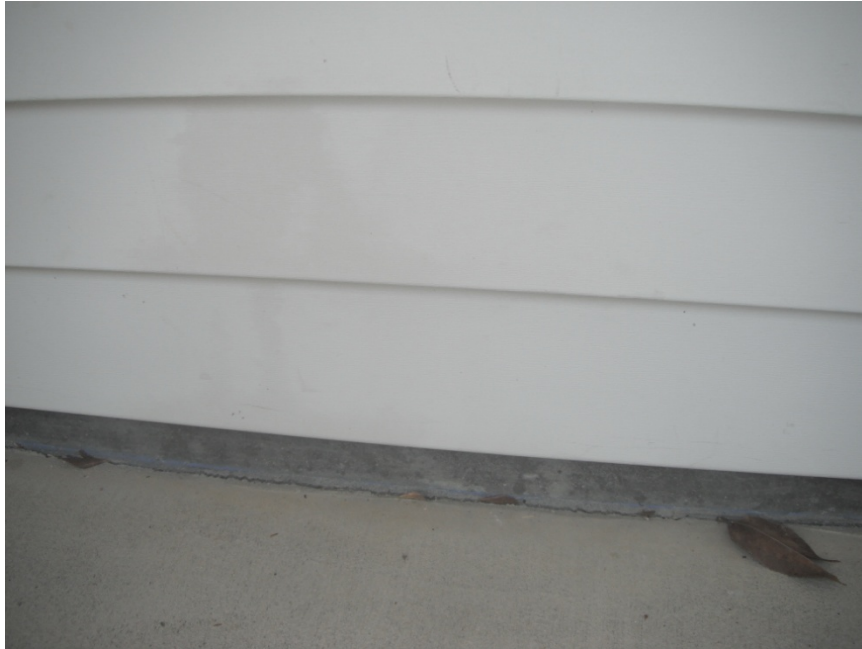
Photograph Number 25 - View of chalk line along front porch – slab settlement.
