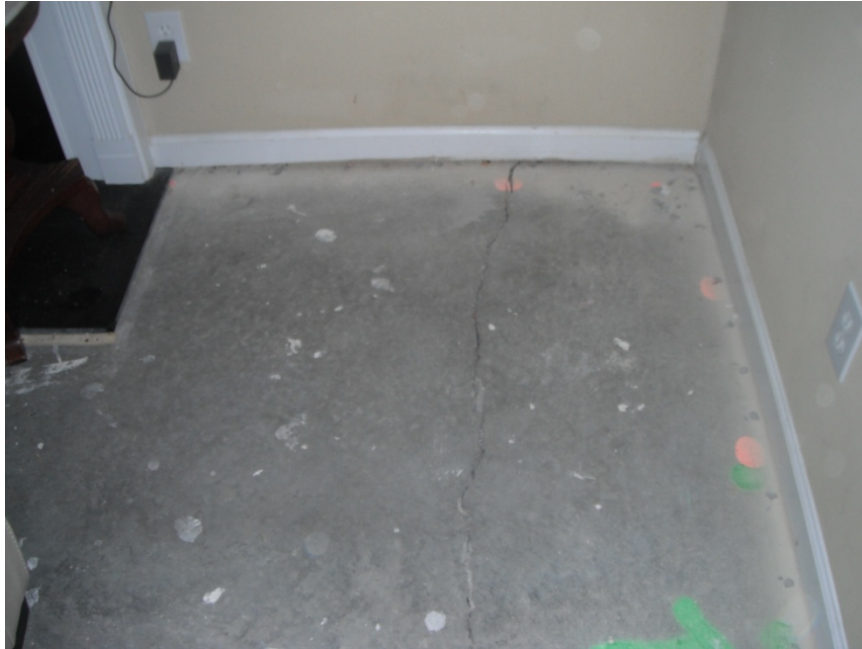
Photograph Number 13 - View of slab cracking.
