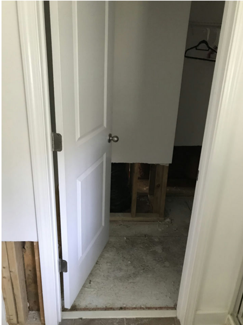
47 Upstairs/Master W.C.2 - 55-W.C (1) Date Taken: 7/1/2019
