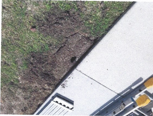
Picture 4 – Example of new footing along back perimeter of proposed screened porch addition
