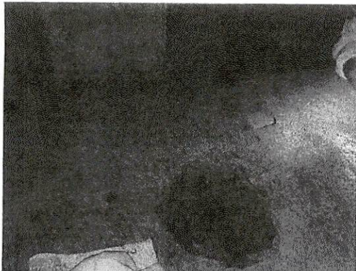
Picture 15 – Example of hole in crawlspace soils, possibly from organic void
