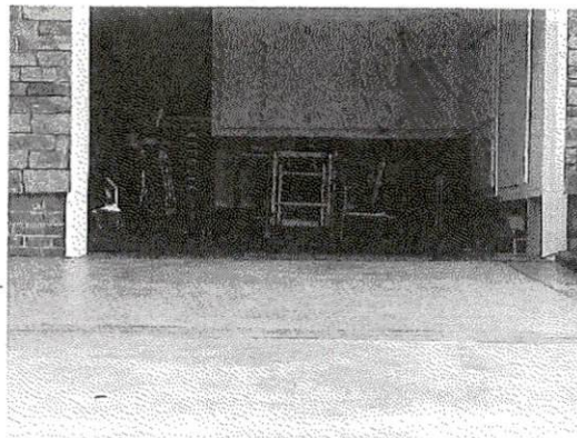
Picture 16 – Example of cracked and settled garage slab
