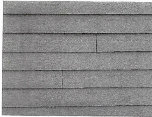
Picture 2 – Example of gaps in siding along garage
