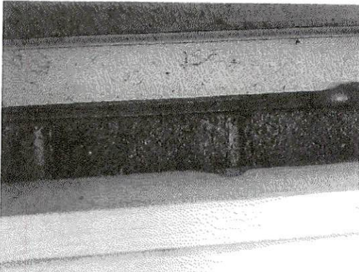
Picture 3 – Example of gap between sill plate and foundation wall
