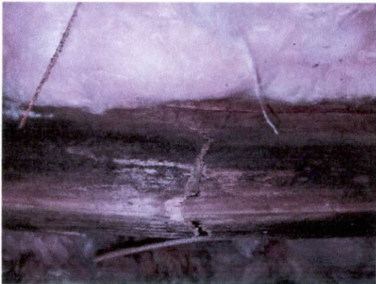
Picture 3 – Example of deteriorated and broken floor joist
