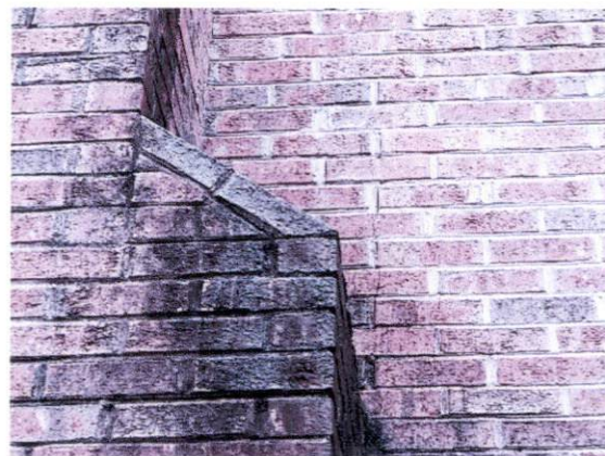
Picture 10 – Example of brick crack along back face of chimney at right wall of home, and water staining on brick face
