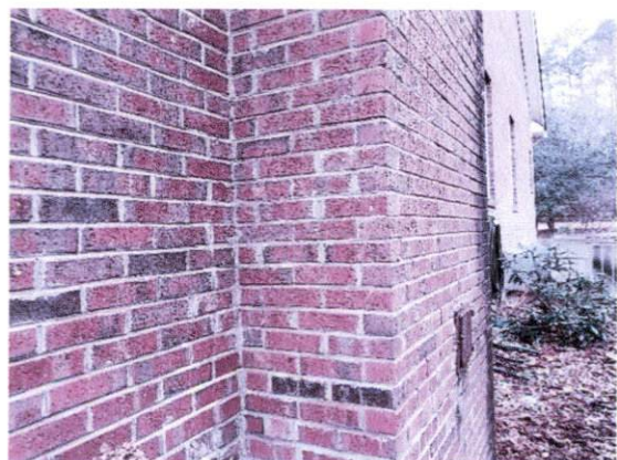
Picture 12 – Example of front face of chimney and right wall of home with no cracks
