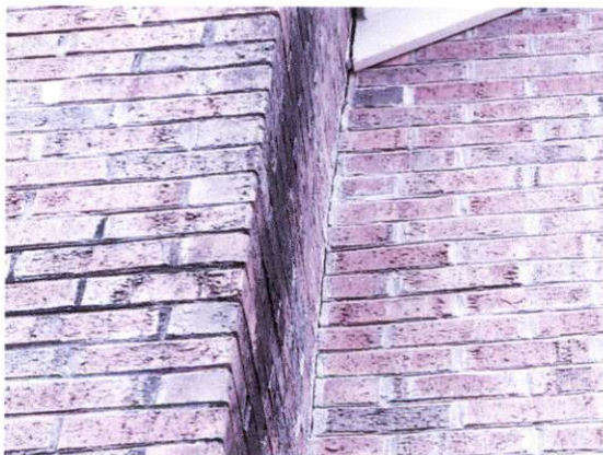
Picture 11 – Example of gap between chimney and end of fly rafter, and brick veneer crack
