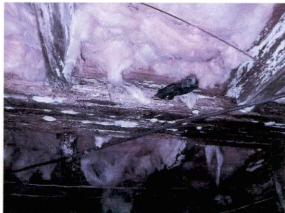
Picture 4 – Example of deteriorated and failed ledger strip
