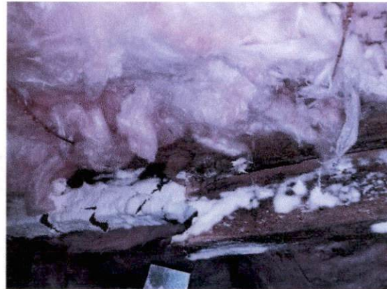
Picture 2 – Example of deteriorated and broken floor joist
