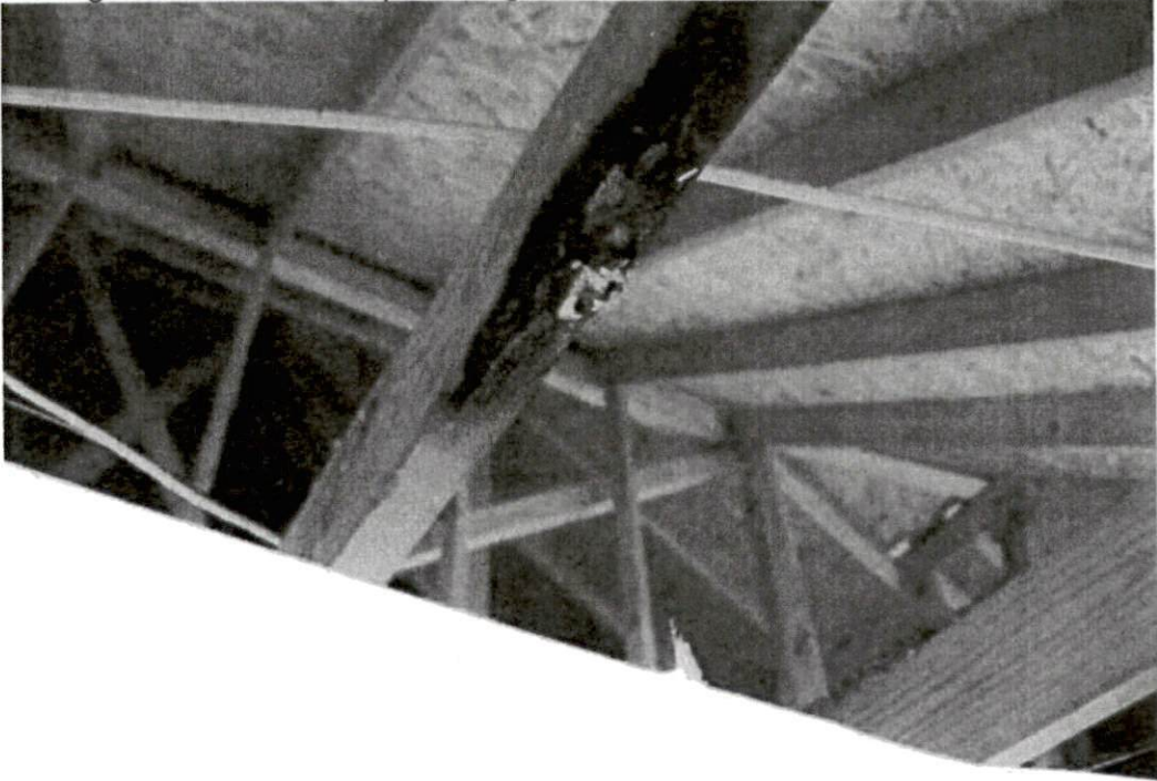
Damage to truss closes to point of ignition
