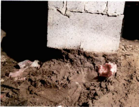
Picture 7 – Example of undermined and inadequately sized piers
