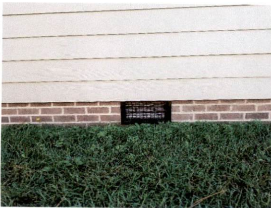
Picture 5 – Example of vent with less than 4" to top of exterior grade
