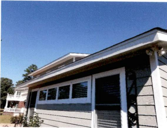
Picture 3 – Example of missing roof gutters
