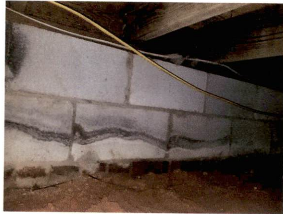
Picture 2 – Example of evidence of water intrusion into crawlspace
