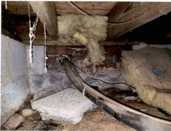
Picture 9 – Inadequately supported joists over foundation wall penetration
