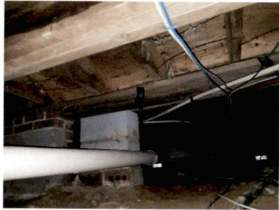
Picture 8 – Inadequately supported joists over foundation wall penetration
