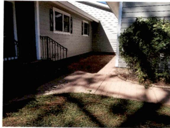
Picture 4 – Example of inadequately sloped exterior grade
