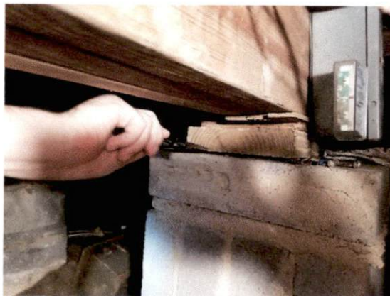
Picture 11 – Example of out-of-contact masonry support
