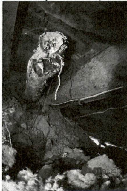
Photograph No. 22 – A root that extended well under the floor framing.
