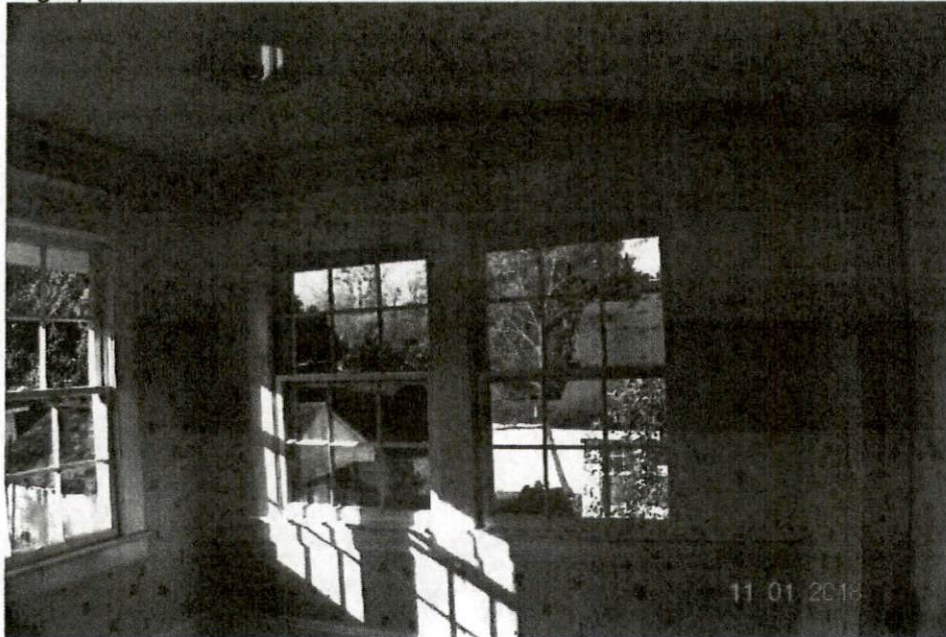
Photograph No. 16 – The room immediately above went along for the ride and shows some distress...
