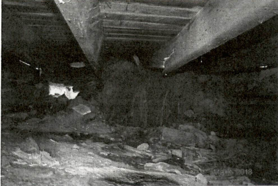
Photograph No. 21 – The only damaged framing member observed is this floor joists above the tree stump. There may be other framing members damaged but they are not visible at this time. We cannot see the sill beam beyond the stump and this may be damaged.
