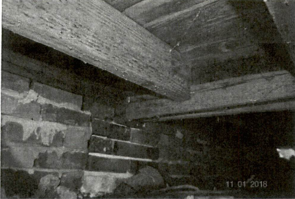
Photograph No. 19 – The pier supporting the left-to-right girder on the left wall is in good shape...
