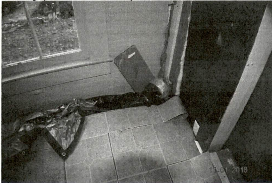
Photograph No. 14 – The rear wall is pushed out a bit.
