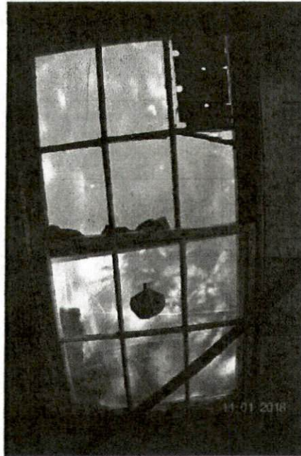
Photograph No. 15 – This window on the left side at the left rear corner is wracked.
