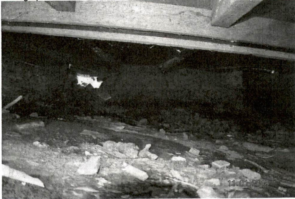
Photograph No. 18 – Looking from the crawlspace under to the rear, showing the root ball.
