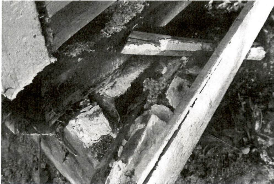
Photograph No. 6 – The left corner pier is damaged. Note the sill beam.
