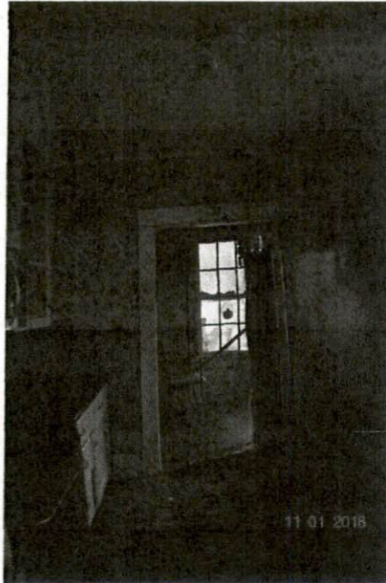
Photograph No. 11 – The kitchen is on the right side of the rear wall, and the hallway is on the left. This photo looks from the kitchen to the hallway. Note the uplift in the hallway floor.
