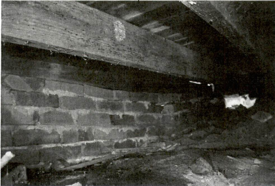
Photograph No. 20 – ... but the face wall is not. The face wall is not a structural component.
