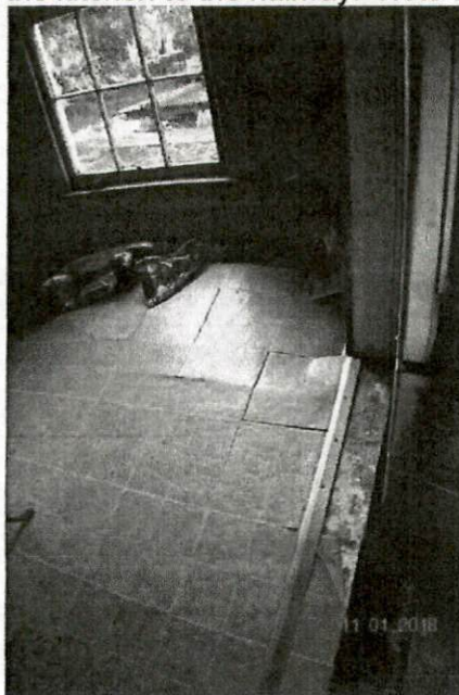
Photograph No. 12 – The stump is right underneath this hallway.
