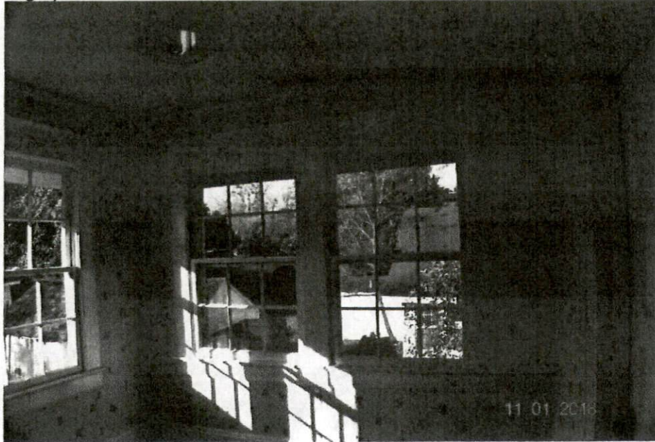
Photograph No. 16 – The room immediately above went along for the ride and shows some distress...
