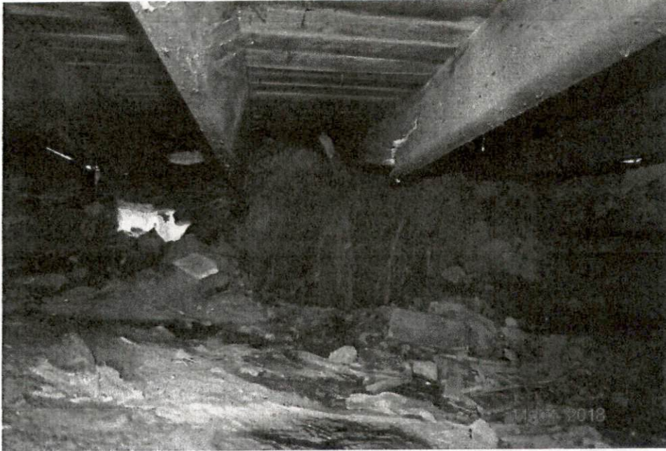
Photograph No. 21 – The only damaged framing member observed is this floor joists above the tree stump. There may be other framing members damaged but they are not visible at this time. We cannot see the sill beam beyond the stump and this may be damaged.
