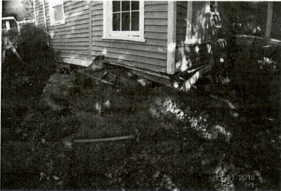
Photograph No. 3 – This is the left rear corner of the home. The tree fell toward the left in this photo, uplifting the left rear corner of the home.
