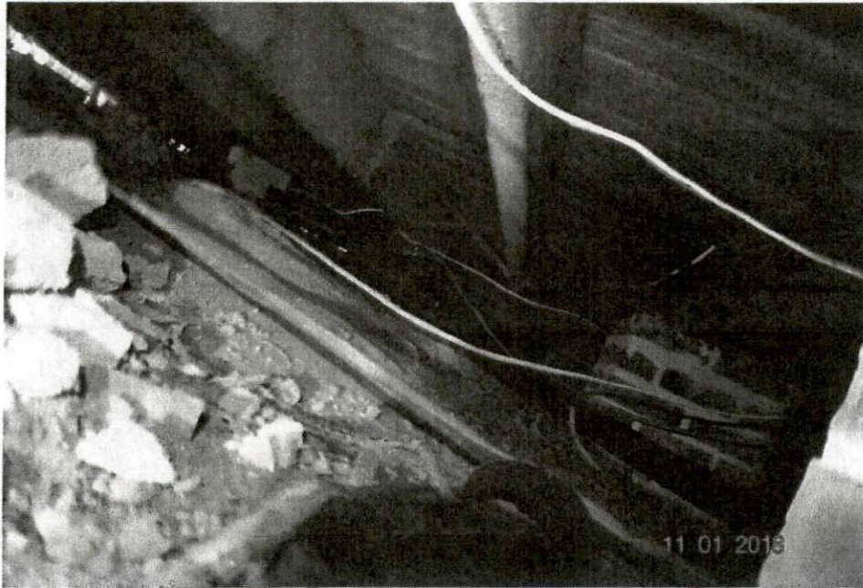
Photograph No. 23 – This photo is taken looking under the kitchen from the left toward the right rear corner. The framing under the kitchen appears undamaged.
