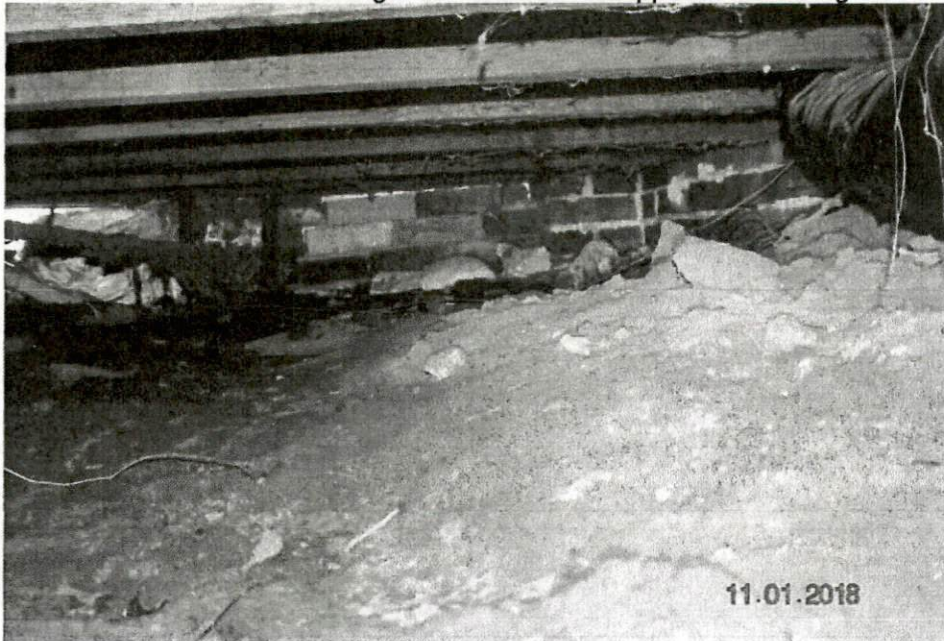
Photograph No. 24 – This photo is taken from the front looking to the right side of the rear wall. The face wall along the rear is damaged.
