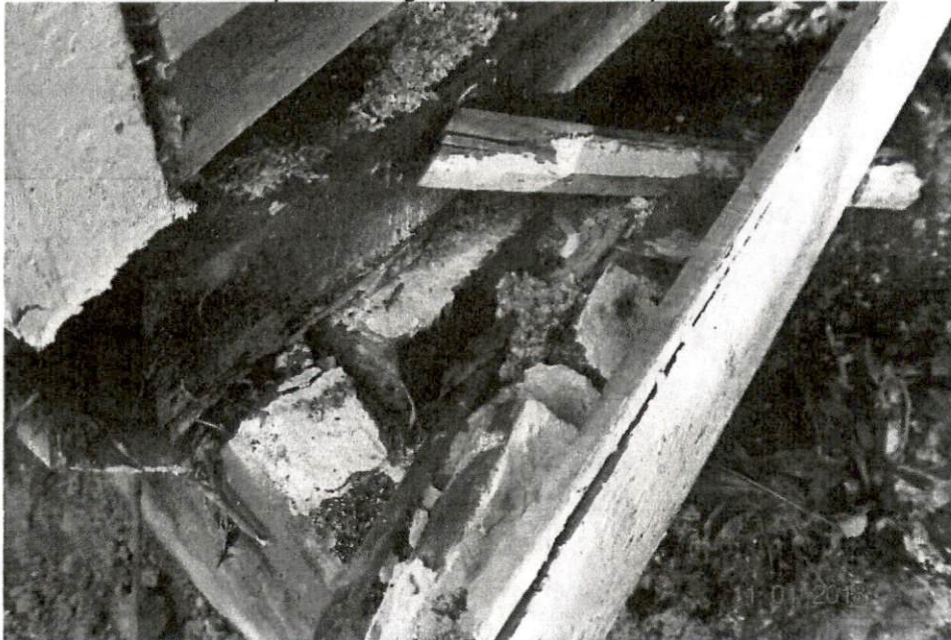
Photograph No. 6 – The left corner pier is damaged. Note the sill beam.
