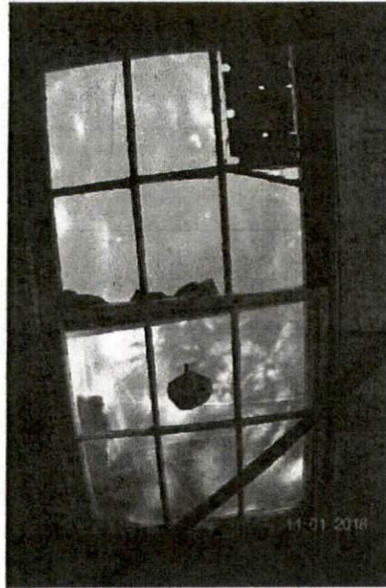
Photograph No. 15 – This window on the left side at the left rear corner is wracked.
