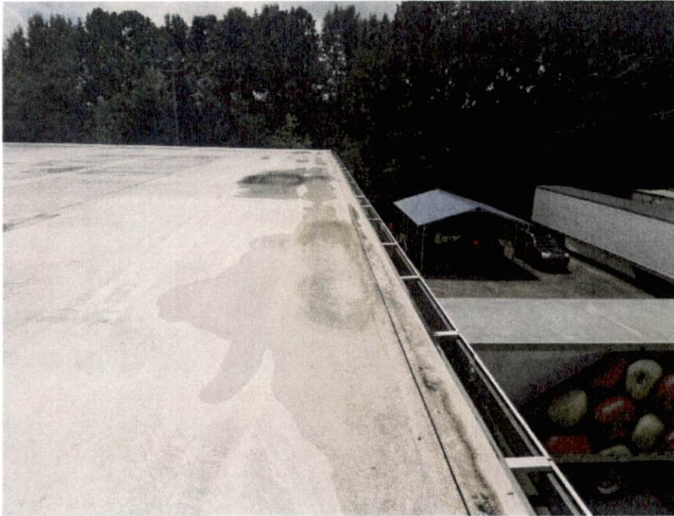
Existing Safety Condition
