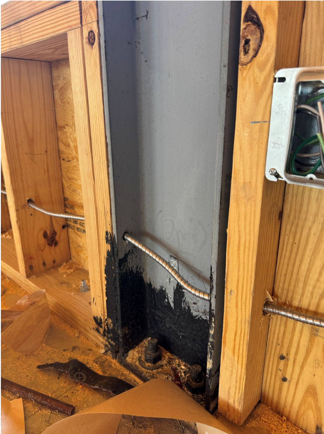
(Conduit Penetration Through Column Flange)
