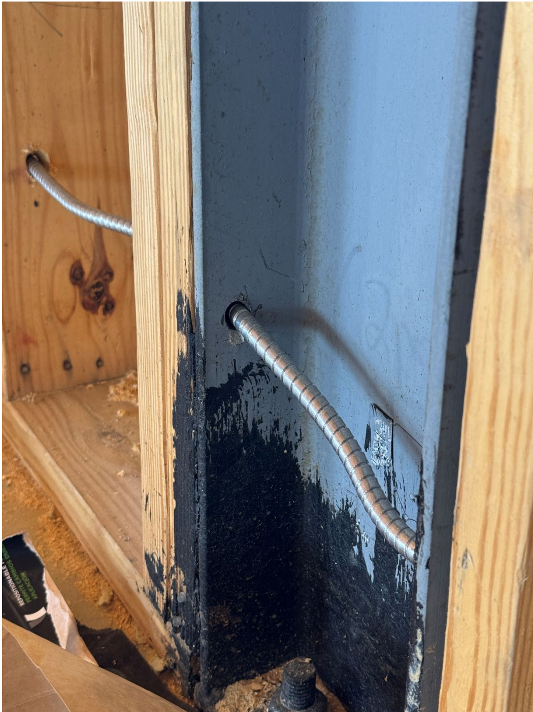
(Conduit Penetration Through Column Flange)
