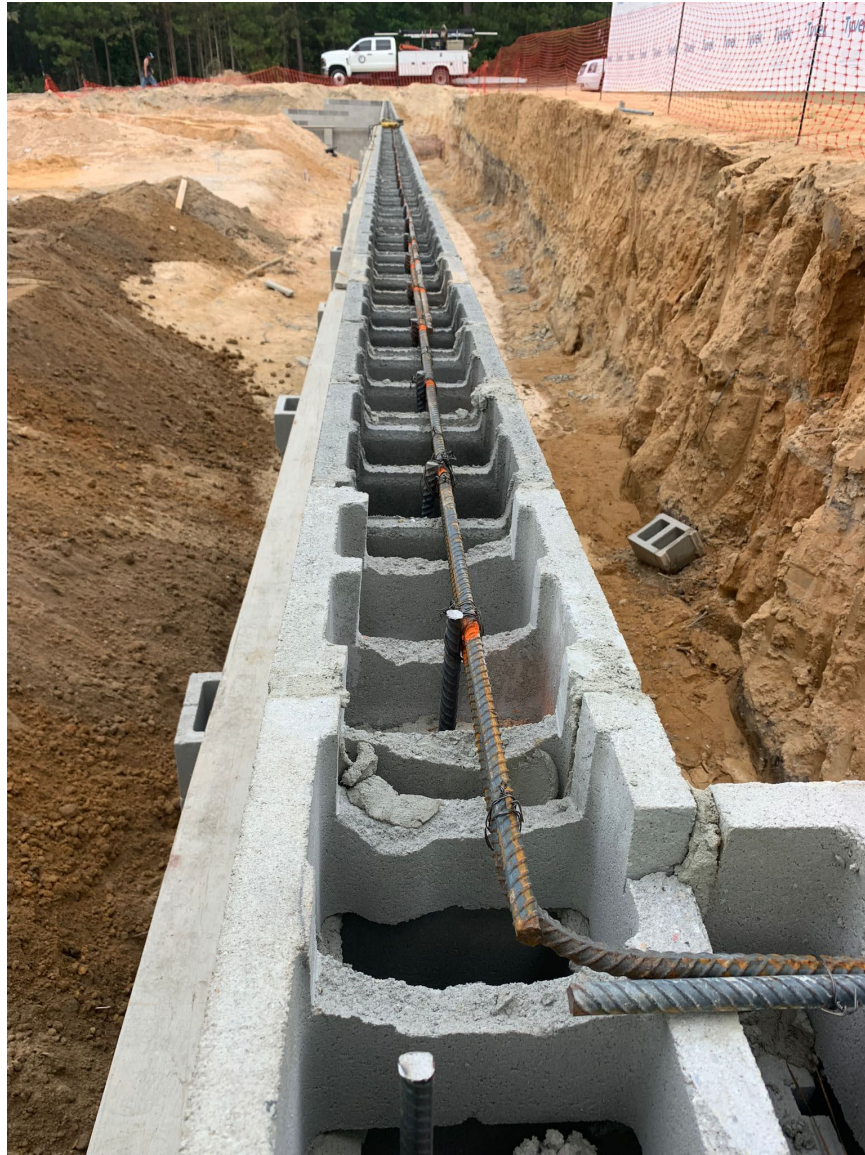
Example of vertical rebar in wall and horizontal rebar at top of wall
