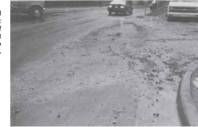
Figure 6.06d Trouble point: Inadequate runoff control—sediment washes onto public road.
