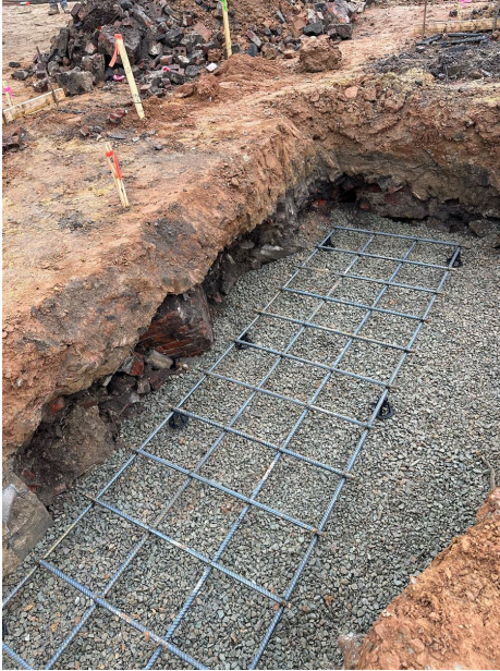
Debris left in place at SW corner, outside the building pad.
