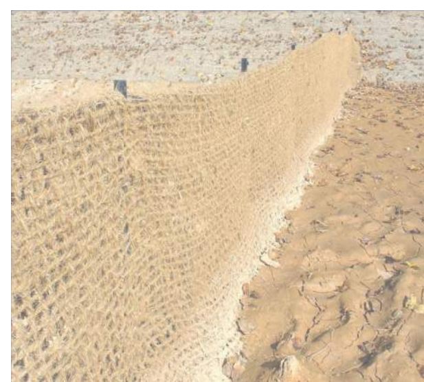
Figure 6.65d Close-up of a porous baffle.
