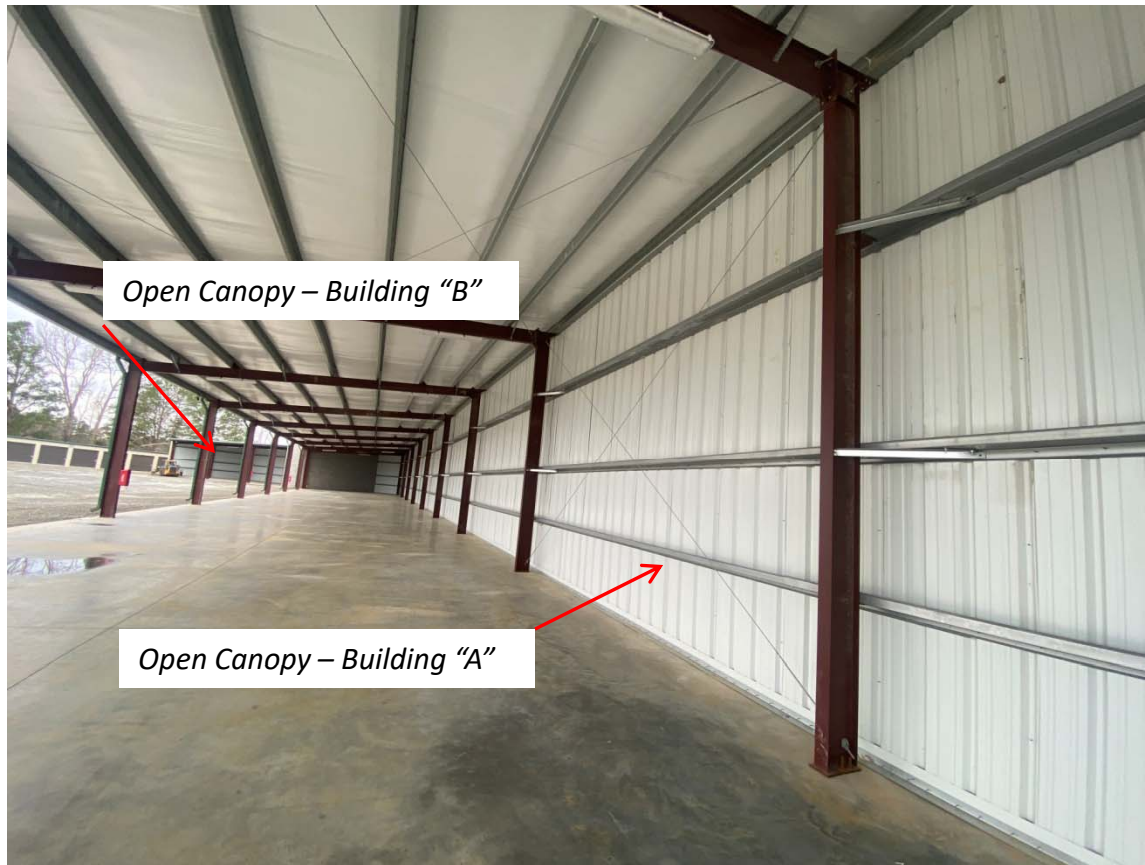
Figure 2 Lakeside Storage Approximate Construction Phase Illustration Buildings "A" & "B" Open Canopy Buildings
