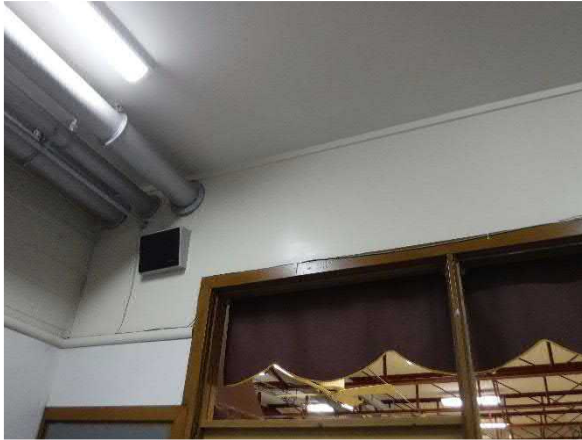
Photo #13 Non-asbestos Plaster Wall and Ceiling (HA #9) above FRP w/Non-Asbestos Glue (HA #10)
