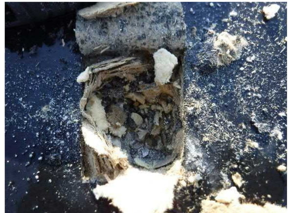
Photo #24 Non-asbestos Black Tar on Foam Insulation (HA #24) and White Gypsum Roof Deck (HA #25)
