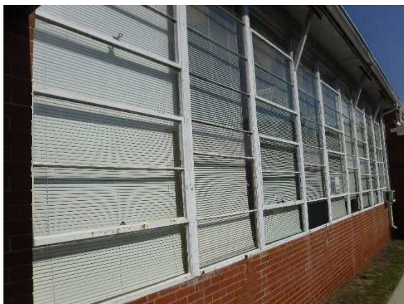
Photo #5 Windows w/Asbestos-Containing Window Glazing (HA #31)
