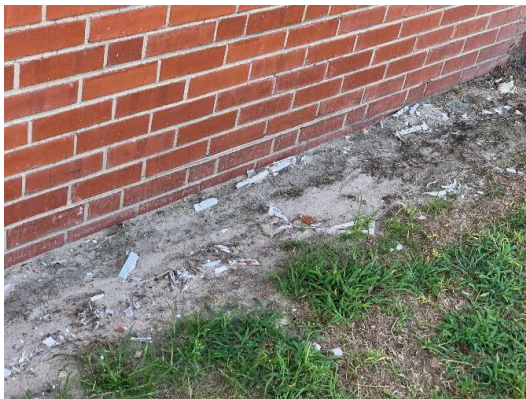
Photo #3 Damaged asbestos-containing window glazing (HA #2) on ground
