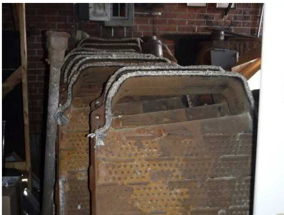
Photo #17 Non-asbestos Boiler Rope Gasket (HA #14)
