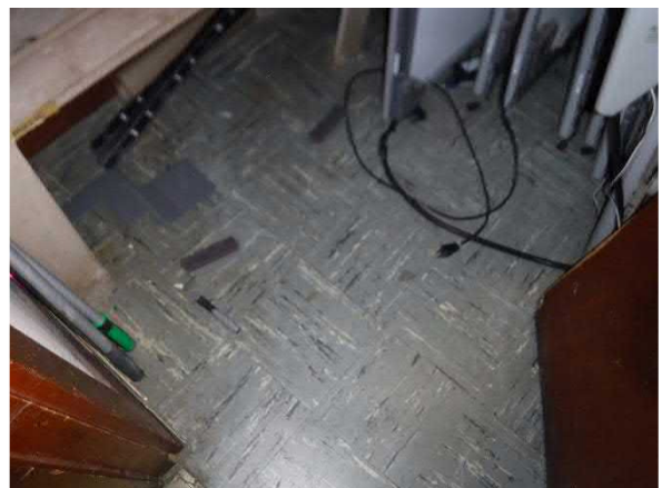
Photo #6 Asbestos-Containing 9"x9" Grey Floor Tile w/White and Grey Streaks/Mastic (previously identified as ACM)
