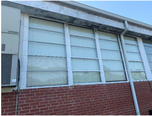
Photo #1 Typical view of windows with asbestos-containing glazing
