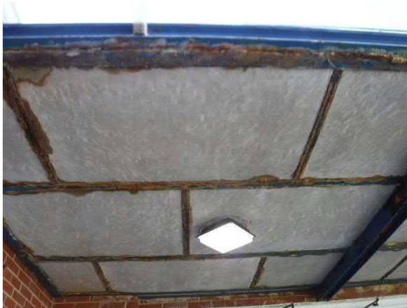
Photo #7 Asbestos-Containing Cementitious Ceiling Panels (previously identified as ACM)
