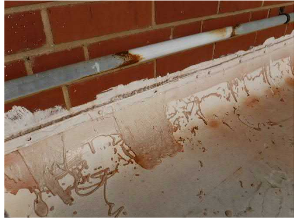
Photo #26 Non-asbestos White Mastic on Roof Flashing (HA #27)
