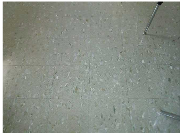
Photo #2 Asbestos-Containing 12"x12" Tan w/Green and Brown Rock Pattern Floor Tile/Mastic (HA #17)
