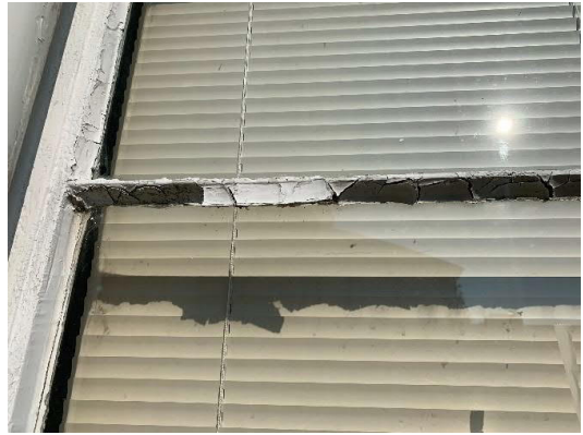
Photo #2 Damaged asbestos-containing window glazing (HA #2)
