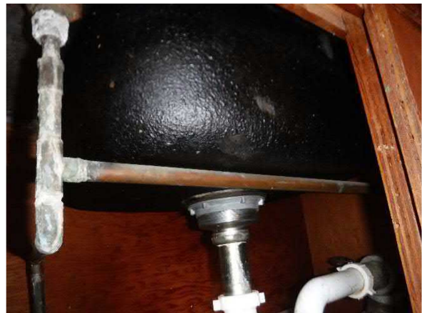
Photo #4 Asbestos-Containing Black Sink Coating (HA #28)
