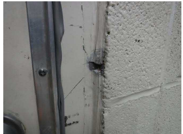
Photo #16 Non-asbestos CMU Block Filler (HA #1) and Grey Interior Door Caulk (HA #13)
