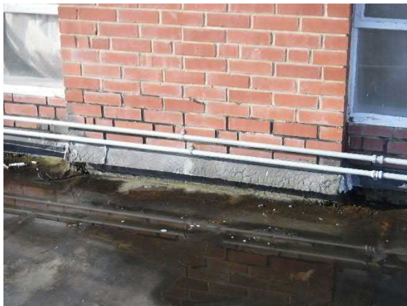
Photo #3 Asbestos-Containing Black Roof Mastic (HA #23)
