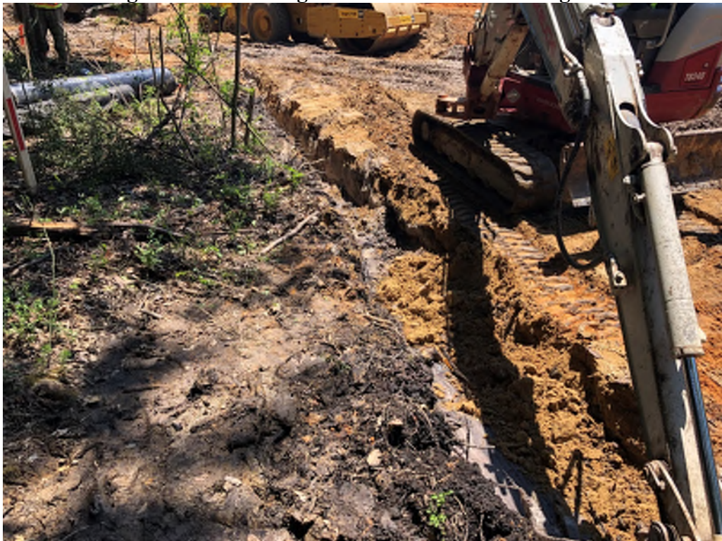
Figure 5: The mini excavator removes wet soil and slough prior to ABC Stone placement
