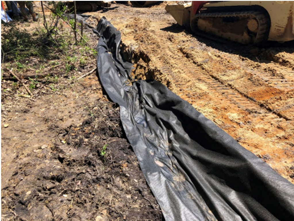
Figure 6: Nonwoven geotextile is placed over the footing subgrade prior to ABC Stone
