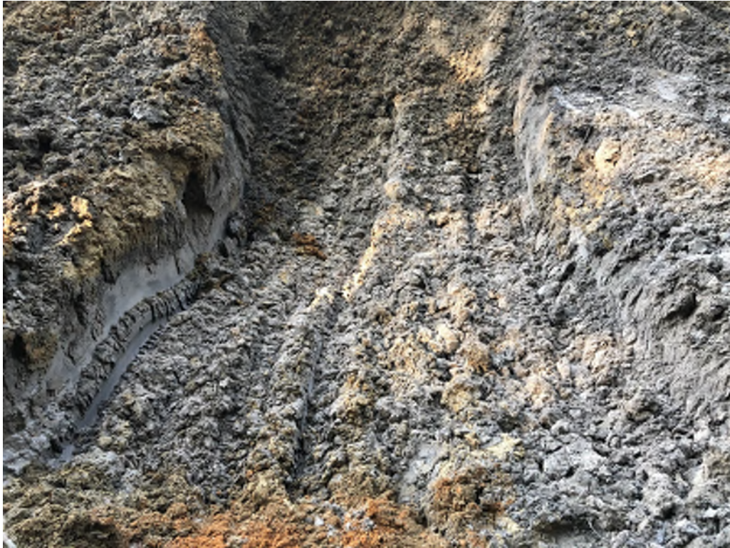
Figure 2: Undercut area at approximately ST 3+50
