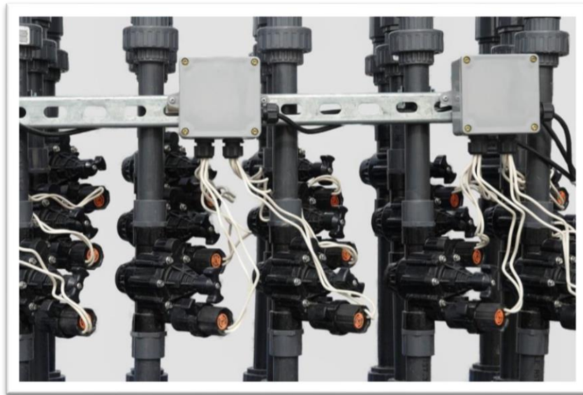
Waterplay manifold – wiring to junction boxes by others
