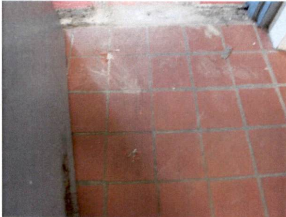
Photo #25 View of HA 21, non-asbestos containing ceramic tile grout and mortar.
