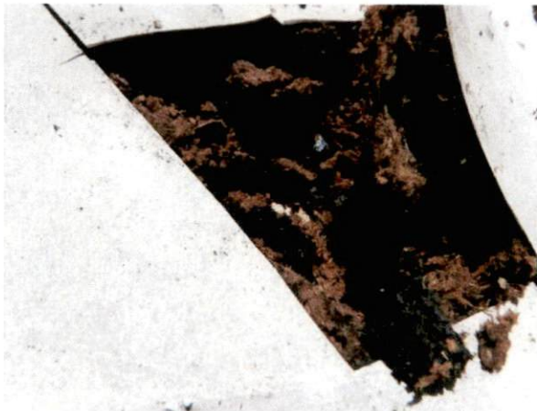
Photo #13 View of HA 6, non-asbestos containing white mastic on EPDM over built-up roofing on west roof.
