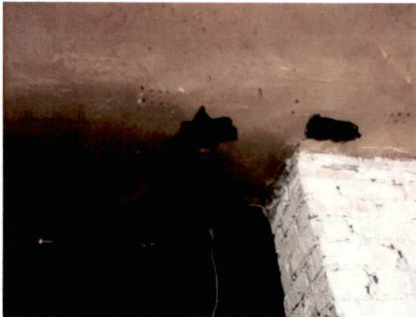
Photo #27 View of HA 23, non-asbestos containing plaster in boiler room.
