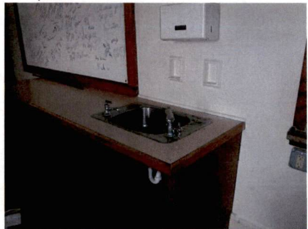
Photo #34 View of sink with HA 29, asbestos-containing black sink mastic.
