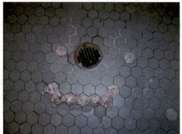
Photo #12 View of HA 5, non-asbestos containing ceramic floor tile grout and mortar.
