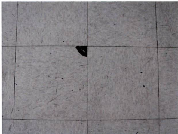
Photo #19 View of HA 13, asbestos-containing mastic associated with non-asbestos containing 12" x 12" tri-beige floor tile and mastic.
