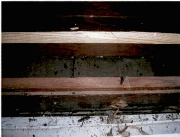
Photo #15 View of HA 9, asbestos-containing 9" x 9" brown floor tile and mastic remaining under built-in shelving.
