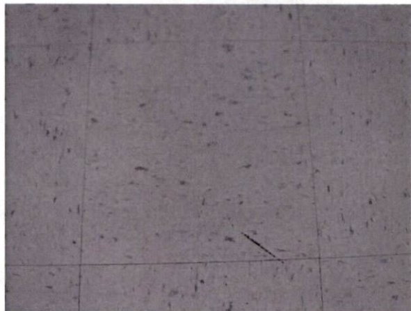
Photo #11 View of HA 4, non-asbestos containing 12" x 12" white with blue and green specks floor tile and mastic.
