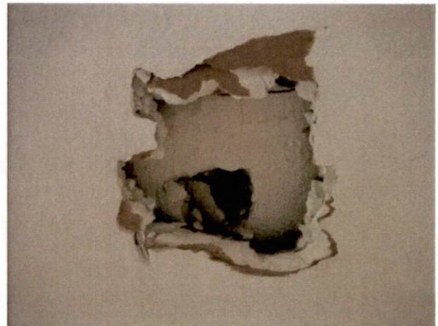
Photo #8 View of HA 2, OSHA-regulated asbestos containing drywall and joint compound over HA 3, non-asbestos containing plaster with drywall lathe.
