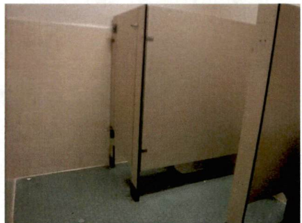
Photo #18 View of HA 12, non-asbestos containing ceramic wall tile grout and mortar.
