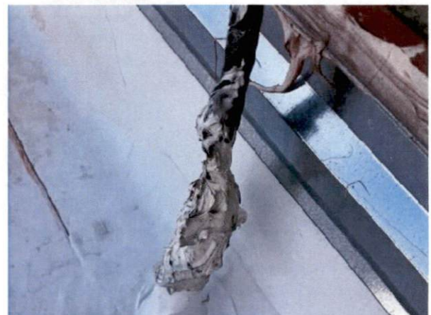
Photo #12 View of HA 5, non-asbestos containing white caulk at lightning rod mount.
