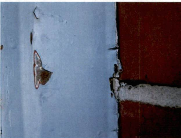
Photo #17 View of HA 10, asbestos-containing beige exterior door caulk.
