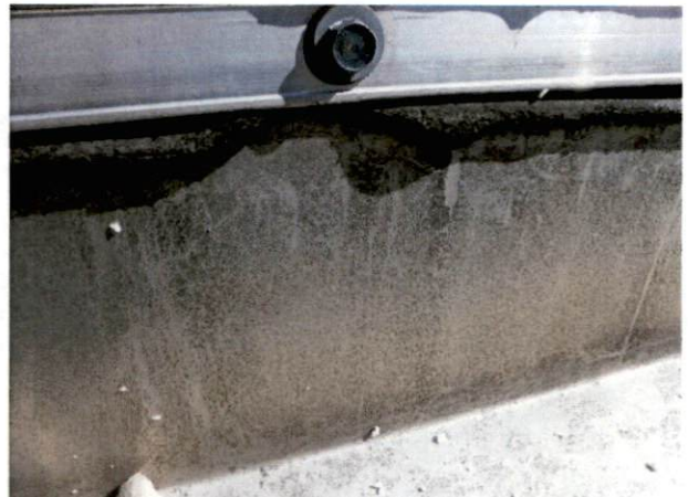
Photo #34 View of HA 30, non-asbestos containing black roof caulk on main roof.
