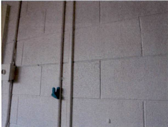
Photo #31 View of HA 25, OSHA-regulated asbestos-containing CMU block filler.
