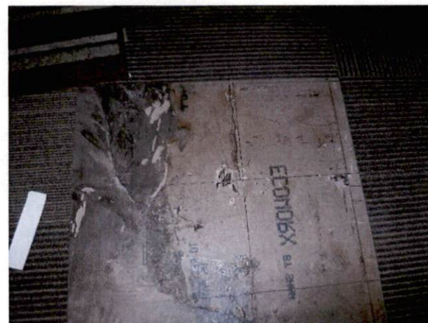
Photo #18 View of HA 14, asbestos-containing 9" x 9" tan floor tile and mastic.
