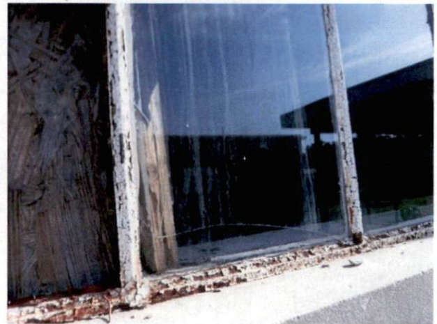
Photo #34 View of HA 28, asbestos-containing exterior window caulk.
