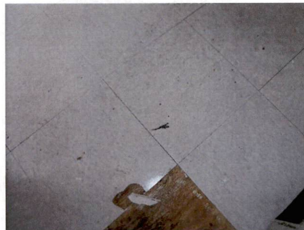
Photo #16 View of HA 12, non-asbestos containing 12" x 12" tri-light gray floor tile and mastic.
