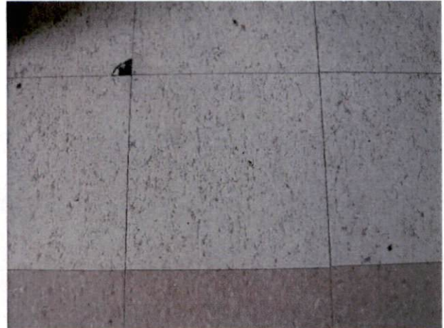
Photo #20 View of HA 14, asbestos-containing mastic with OSHA-regulated asbestos-containing 12" x 12" off-white with brown and white specks floor tile.
