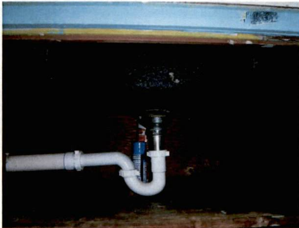
Photo #9 View of HA 4, asbestos-containing black sink mastic.
