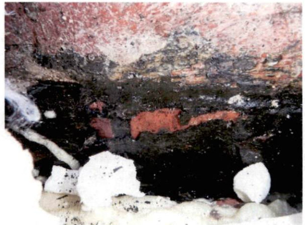
Photo #10 View of HA 3, non-asbestos containing black roof mastic on east roof.
