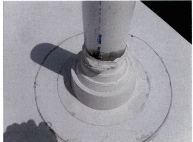
Photo #8 View of HA 2, non-asbestos containing white roof caulk at penetrations on east roof.
