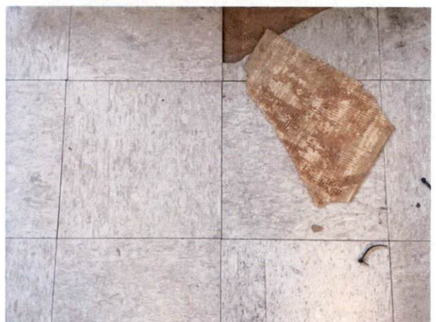
Photo #24 View of HA 20, non-asbestos containing 12" x 12" beige with tan and white splotches floor tile and mastic.
