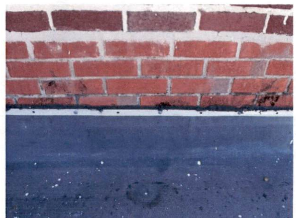
Photo #12 View of HA 5, non-asbestos containing black roof caulk on west roof.
