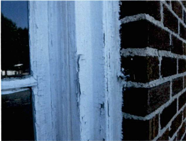
Photo #37 View of HA 33, asbestos containing exterior caulk.
