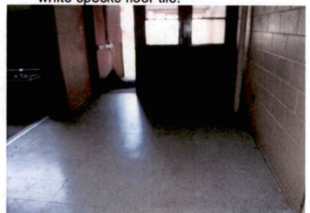
Photo #24 View of HA 20, asbestos-containing mastic with OSHA-regulated asbestos-containing 12" x 12" light gray with white specks floor tile.
