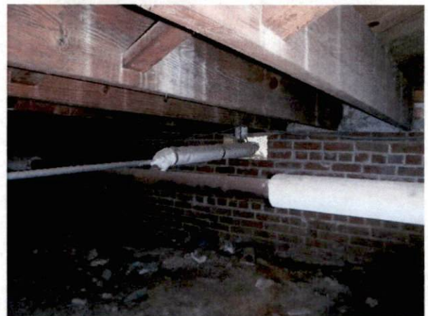
Photo #10 View of crawlspace with HA 1, asbestos-containing air-o-cell pipe insulation and HA 3, asbestos-containing hard TSI joint.
