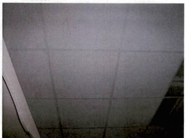
Photo #30 View of HA 23 non-asbestos drywall and joint compound above HA 24, non-asbestos containing ceiling tile.
