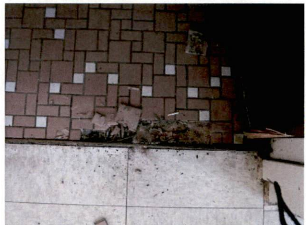
Photo #30 View of HA 24, non-asbestos containing ceramic floor tile grout and mortar.
