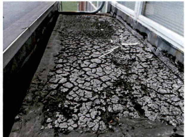
Photo #16 View of HA 10, non-asbestos containing built-up roofing with silver paint on canopy.
