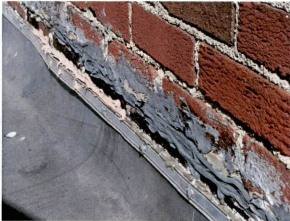
Photo #31 View of HA 27, asbestos containing black roof mastic and non-asbestos containing gray roof mastic.
