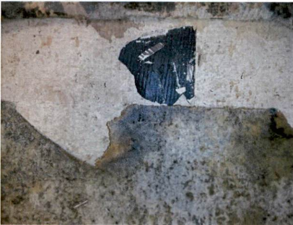
Photo #21 View of HA 17, asbestos-containing 12" x 12" tan with brown dots floor tile with non-asbestos containing mastic.
