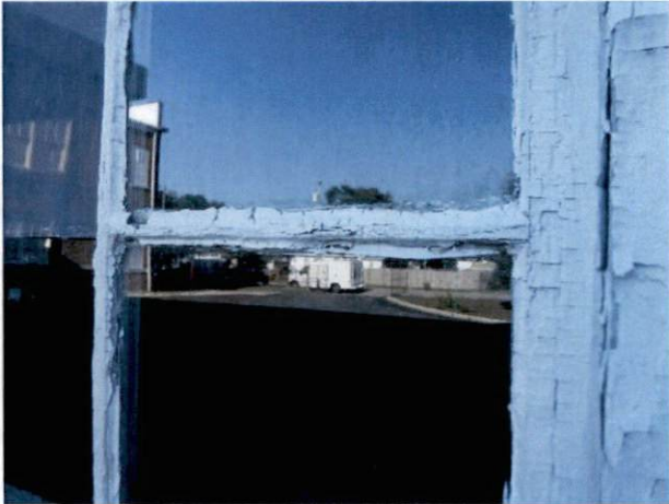
Photo #38 View of HA 34, asbestos containing exterior window glazing.
