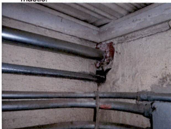
Photo #23 View of HA 17, non-asbestos containing brittle red fire caulk.
