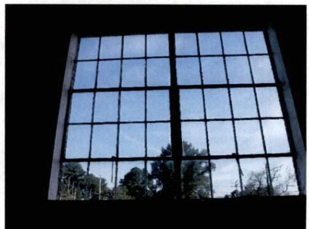
Photo #36 View of HA 32, asbestos-containing white with gray interior window glazing.
