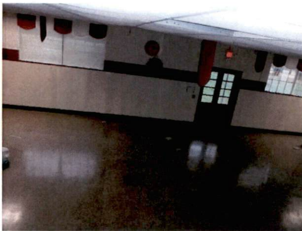
Photo #35 View of cafeteria with HA 29, asbestos-containing interior window glazing.
