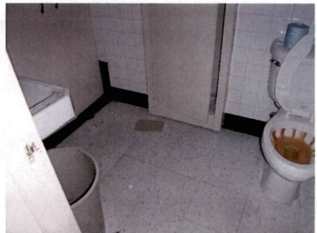
Photo #24 View of HA 16, restroom with non-asbestos containing 12" x 12" light gray with gray specks floor tile and mastic.
