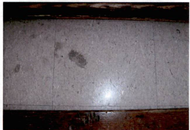
Photo #22 View of HA 18, asbestos-containing mastic with OSHA-regulated asbestos-containing 12" x 12" pink with white specks floor tile.
