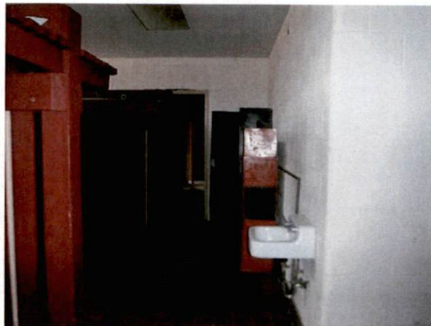
Photo #26 View of boy's locker room with HA 22, non-asbestos containing 2' x 2' white drywall ceiling tile.
