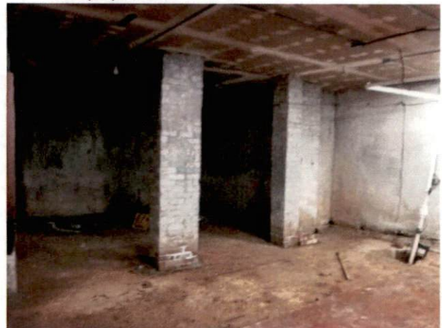
Photo #28 View of boiler room with HA 24, OSHA-regulated asbestos-containing drywall and joint compound in boiler room.
