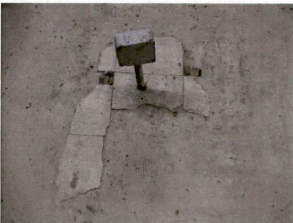
Photo #17 View of HA 9, asbestos-containing 9" x 9" gray floor tile and mastic in basement.
