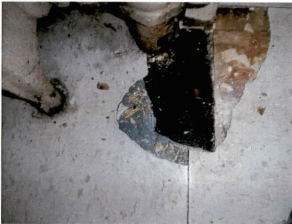
Photo #25 View of HA 17, asbestos-containing tan floor tile and mastic and HA 18, non-asbestos containing blue floor tile with asbestos-containing mastic.
