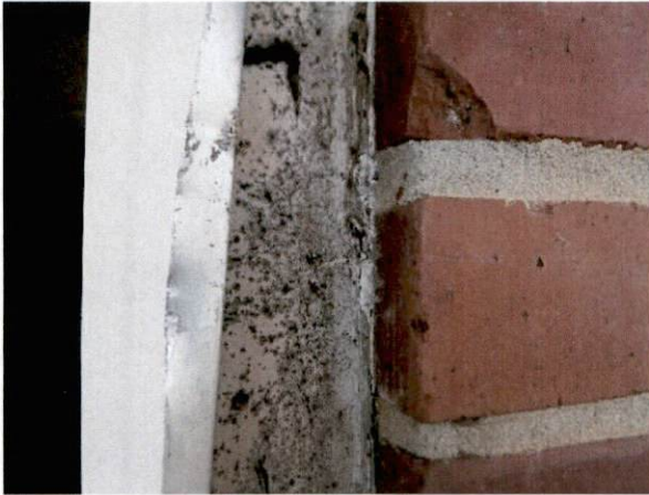
Photo #37 View of HA 32, asbestos-containing exterior caulk.
