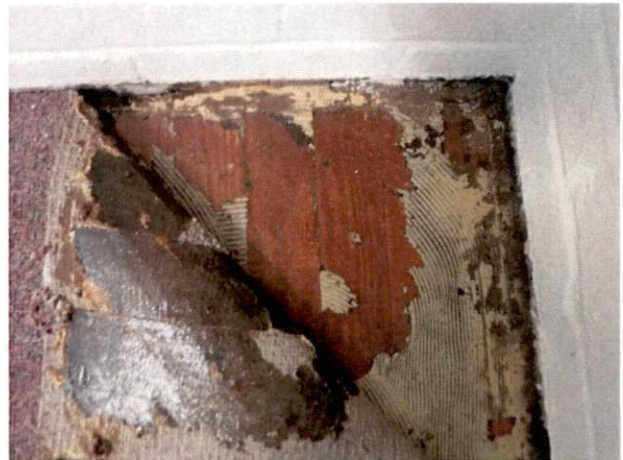
Photo #32 View of HA 26, non-asbestos containing yellow carpet glue and brown paint.
