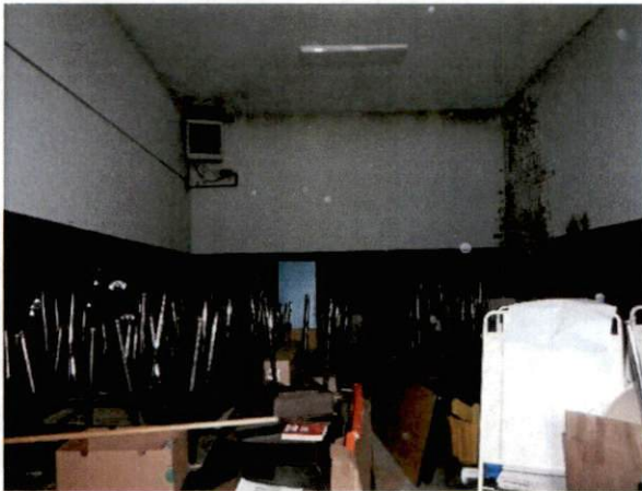
Photo #15 View of storage room with HA 8, non-asbestos containing textured ceiling plaster.
