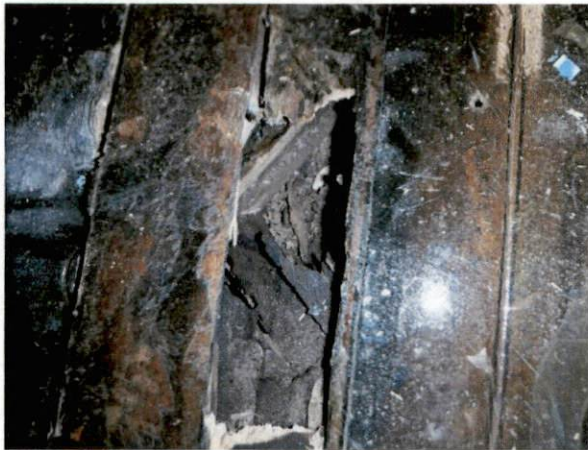
Photo #7 View of HA 1, non-asbestos containing black felt paper under hardwood flooring.
