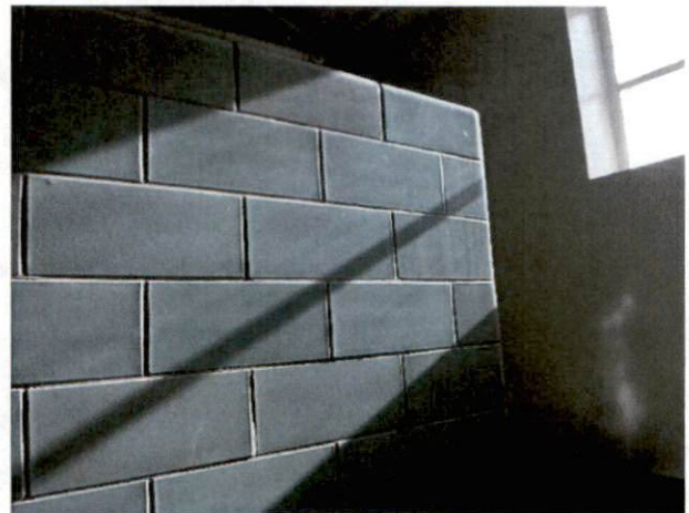
Photo #28 View of HA 22, non-asbestos containing ceramic wall tile grout and mortar.
