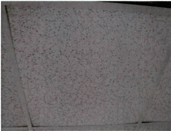
Photo #15 View of HA 8, non-asbestos containing 2' x 2' white ceiling tile with dots and pits.
