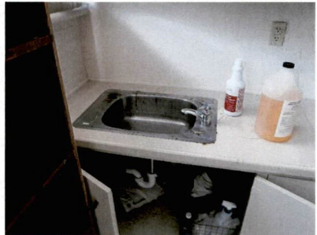
Photo #14 View of sink with HA 8, asbestos-containing black sink mastic.
