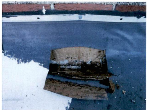
Photo #14 View of HA 7, asbestos-containing silver paint and black flashing on west roof.
