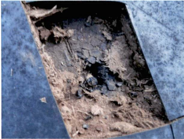
Photo #19 View of HA 12, non-asbestos containing built-up roofing under black membrane on southwest roof.
