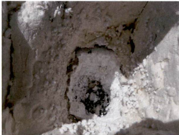
Photo #9 View of HA 2, non-asbestos-containing black tar under roof membrane and foam insulation.
