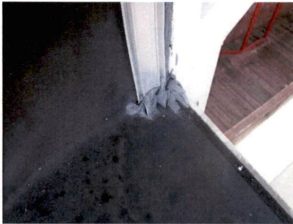
Photo #21 View of HA 13, non-asbestos containing black roof caulk.
