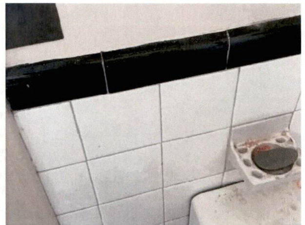
Photo #40 View of HA 36, non-asbestos containing ceramic wall tile grout and mortar.
