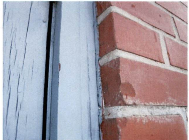
Photo #16 View of door frame with HA 9, asbestos-containing white exterior door caulk.
