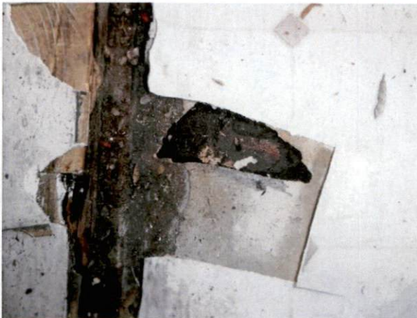
Photo #27 View of HA 20, non-asbestos containing gray vinyl sheet flooring with black felt backing.
