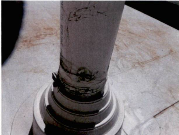
Photo #9 View of HA 2, asbestos-containing white roof caulk at penetrations on west roof.
