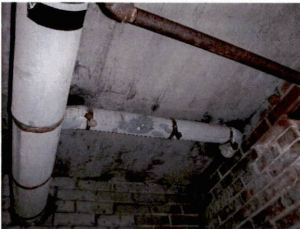
Photo #9 View of HA 3, asbestos-containing hard TSI joint associated with HA 1.
