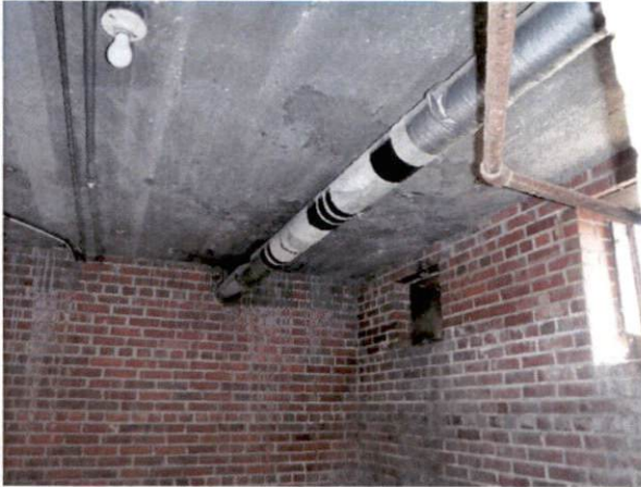
Photo #7 View of HA 1, asbestos-containing air-o-cell pipe insulation.
