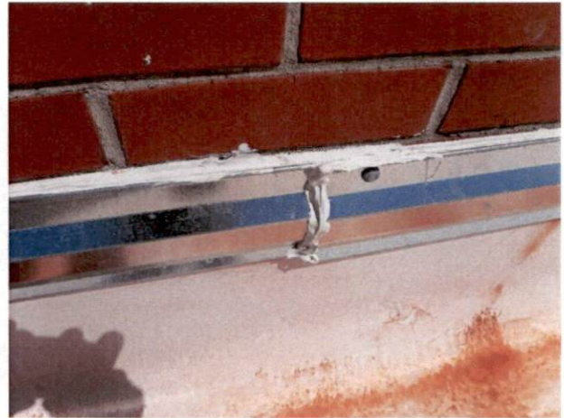
Photo #8 View of HA 1, non-asbestos containing white roof caulk at brick on west roof.
