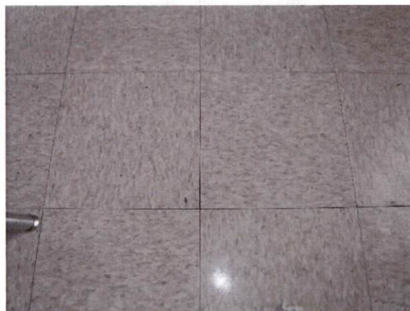
Photo #15 View of HA 11, non-asbestos containing 12" x 12" tri-tan floor tile and mastic.
