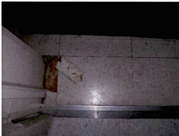
Photo #23 View of HA 15, non-asbestos containing 12" x 12" off-white speckled floor tile and mastic.
