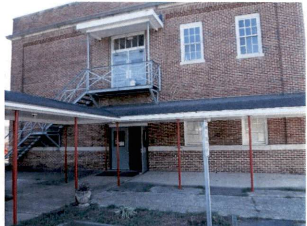
Photo #26 Canopy with HA 22, non-asbestos containing gray/black asphalt shingles and felt paper.
