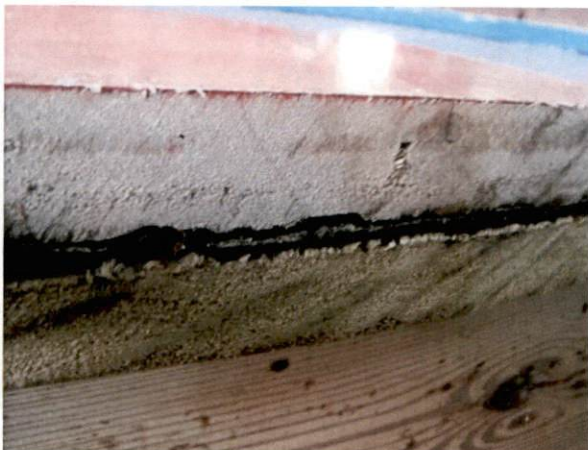
Photo #25 View of HA 21, non-asbestos containing black felt paper under hardwood flooring.
