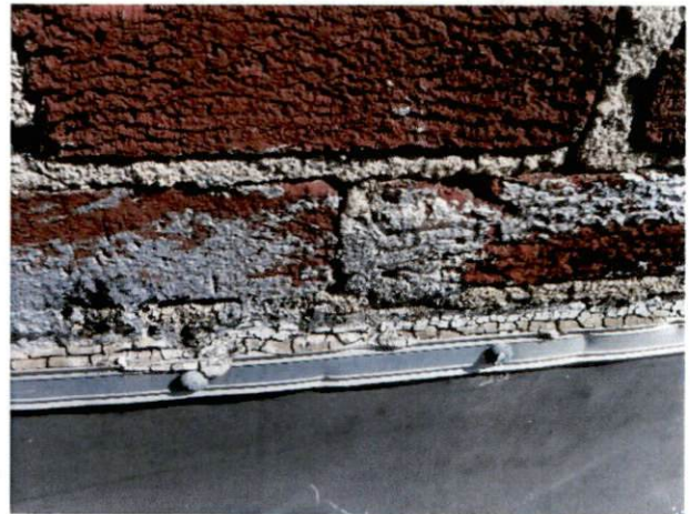
Photo #32 View of HA 28, asbestos-containing silver paint.
