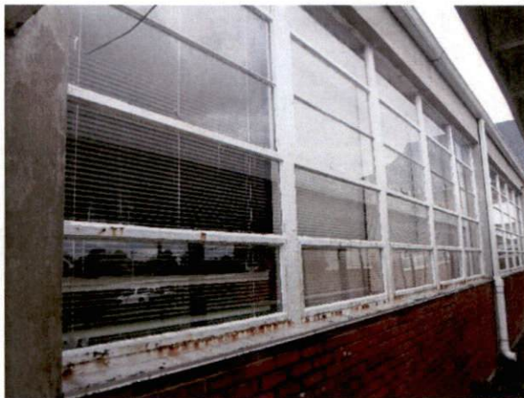
Photo #21 View of windows with HA 15, non-asbestos containing off-white exterior window glazing.
