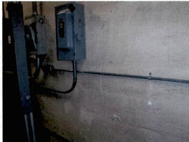
Photo #20 View of HA 14, asbestos-containing textured coating on CMU and brick walls.
