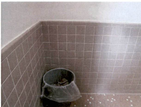
Photo #29 View of HA 23, non-asbestos containing ceramic wall tile grout and mortar.
