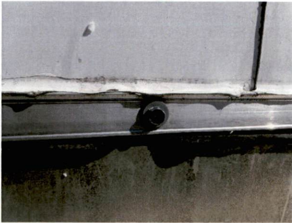
Photo #33 View of HA 29, non-asbestos containing white roof caulk on main roof.
