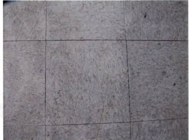
Photo #32 View of HA 26, non-asbestos containing 12" x 12" off-white with brown specks floor tile and mastic.
