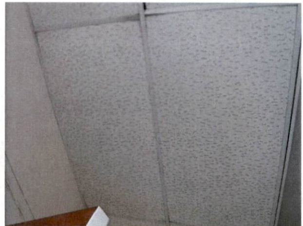
Photo #26 View of HA 20, non-asbestos containing 2' x 4' white ceiling tile with dots and fissures.
